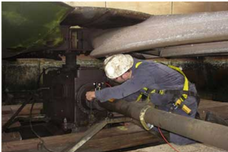
There is not much room under the large fan blades for the apprentice but the other Laser/Detector is mounted on the Gearbox shaft.
